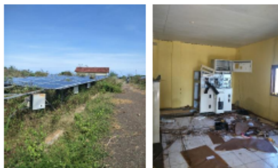
Fig. 9 Current condition of PV arrays and control room of Sumbawa PV plant
