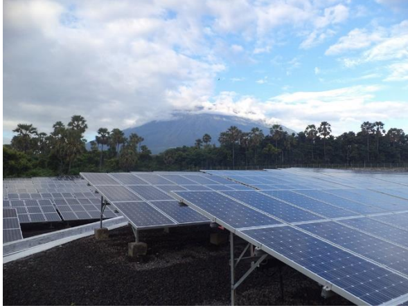
Figure 31 Array of Karangasem PV plant
